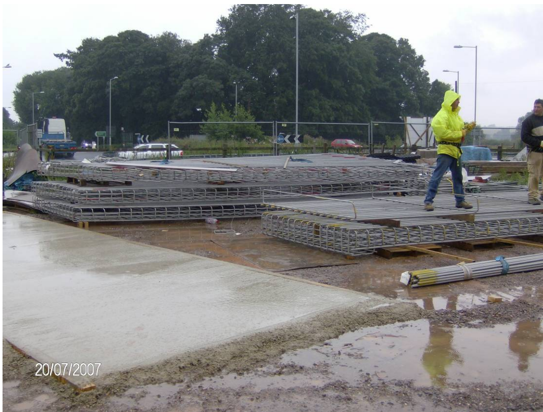
Photograph 5 Casting Operation at Downton Industrial Estate Showing Reinforcement Cages for Bridge Deck Units
