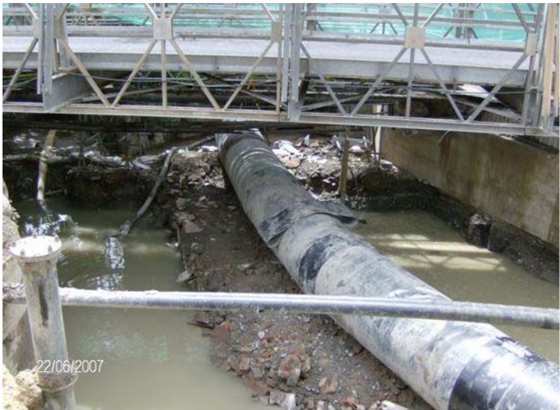
The pipe run to The Corn Mill. The infill concrete adjacent to the "triangular island" is also visible on the right of the photograph.
