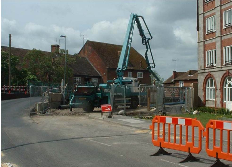
Concrete pump in position for pouring of concrete infill (infill area adjacent to central “island”)
