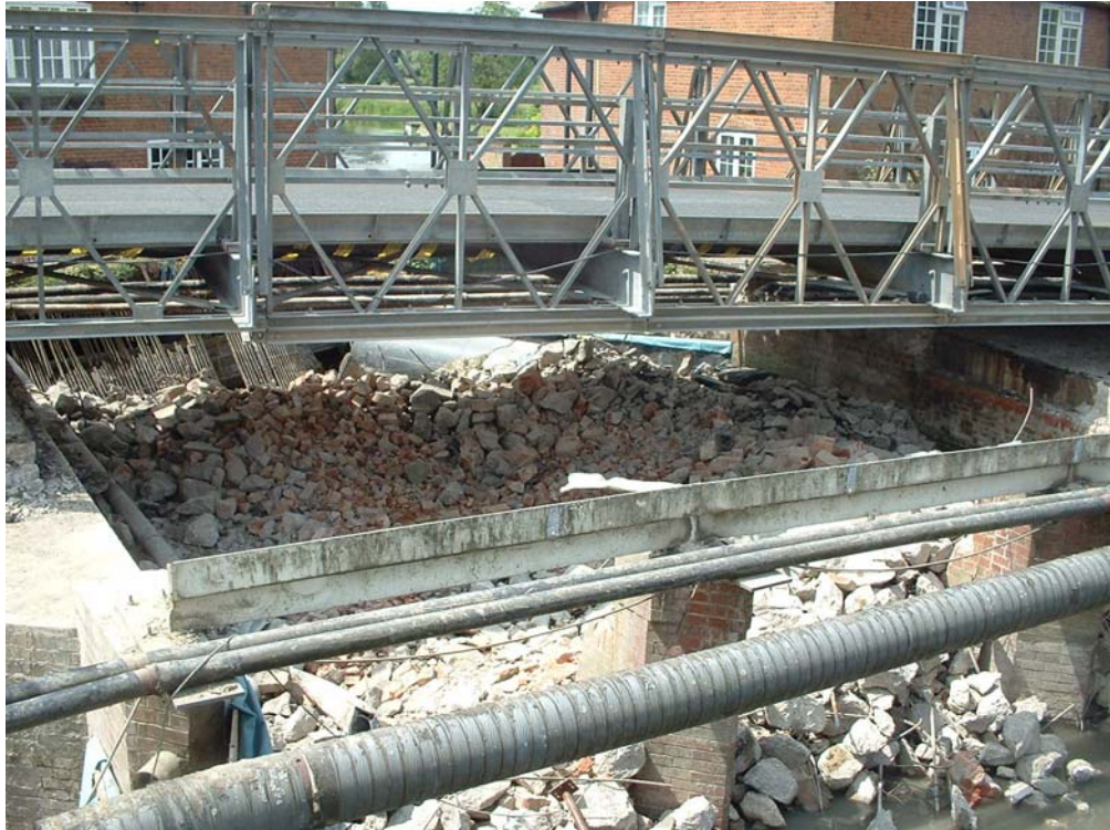
Debris from demolition on West side of central "island" (to be removed)
